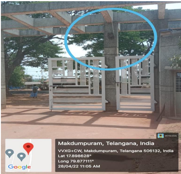
CCTV Camera At College Entrance Gate
